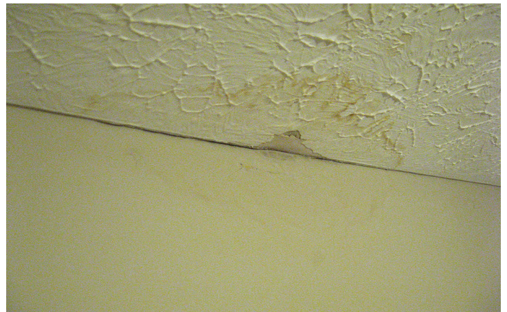
Figure 2: Wrinkled coating due to water damage.
