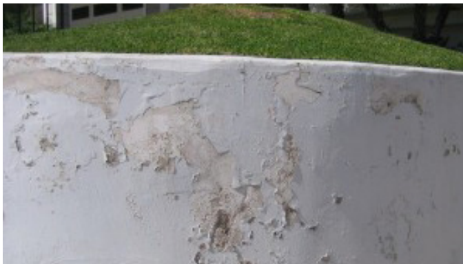
Figure 3: Water damage on stucco wall.
